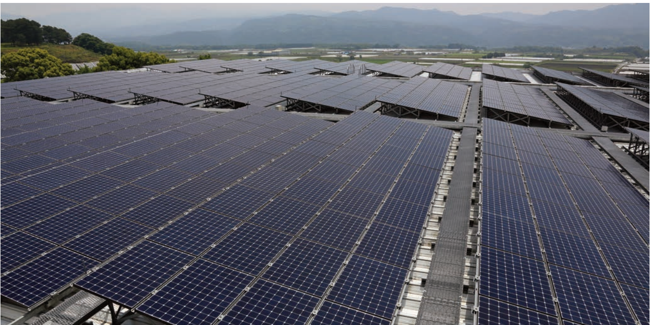
SunPower solar panels, Kumamoto, Japan.
