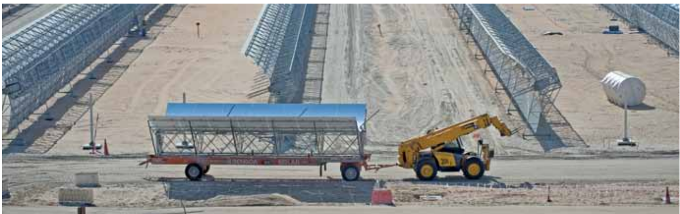
Solar power plant in Madinat Zayed, United Arab Emirates.
